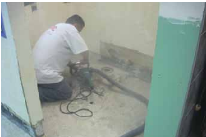
ABOVE ▲ “The floor that we were working on was on the second floor of the mortuary — directly above a client area — so it had to be absolutely watertight,” says Tabrizi.
