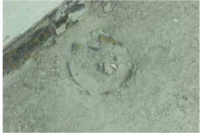
ABOVE ▲ “As we exposed the slab we uncovered an old set of unused pipes that given — the age, setting, and possible use — had to be removed by the mortuary,” explains Tabrizi.
